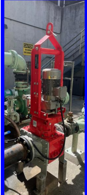
New Secondary Grinder
