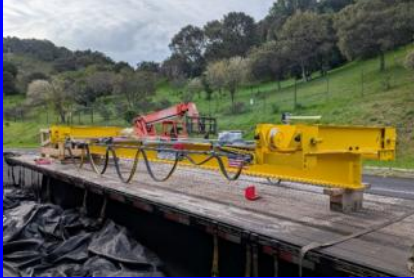
New Bridge Crane
